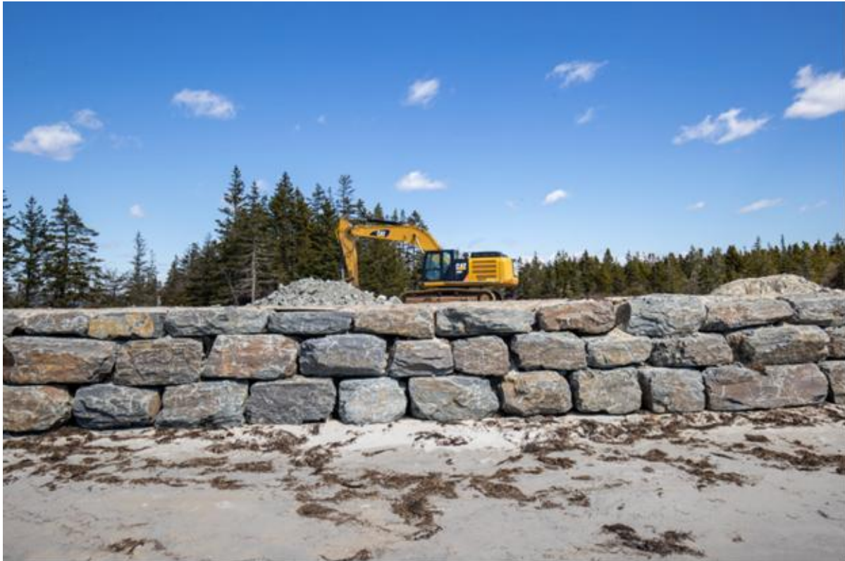
Seawall being constructed at Little Crescent Beach, La Have region, Lunenburg County. Nicolas Winkler Photography (2024).
